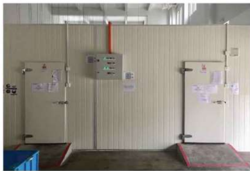
Walk In Chiller ( 0 - 4°C ) x 2 rooms
